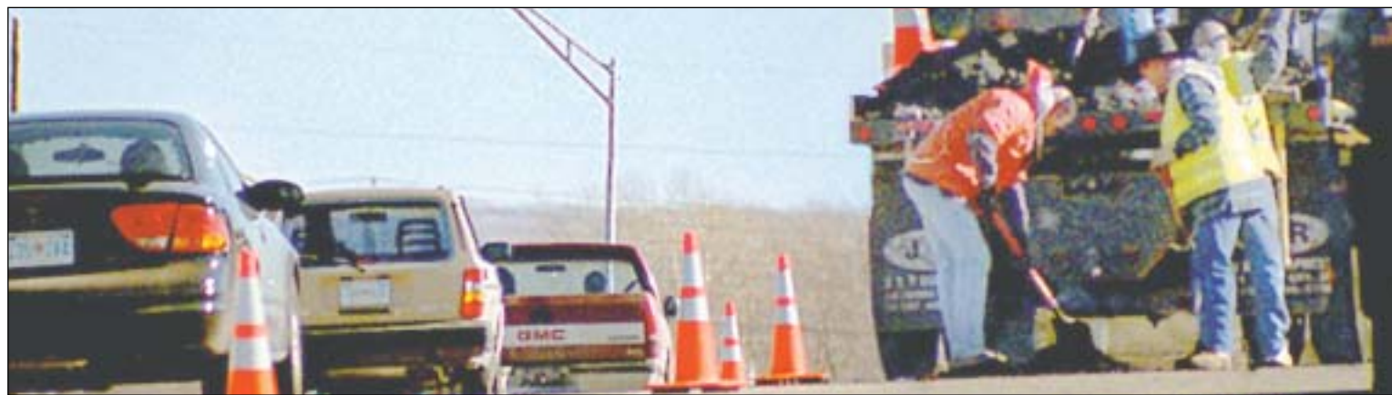
Oklahoma Department of Transportation workers repair a pothole on the Broken Arrow Expressway near the Sheridan Road exit.
